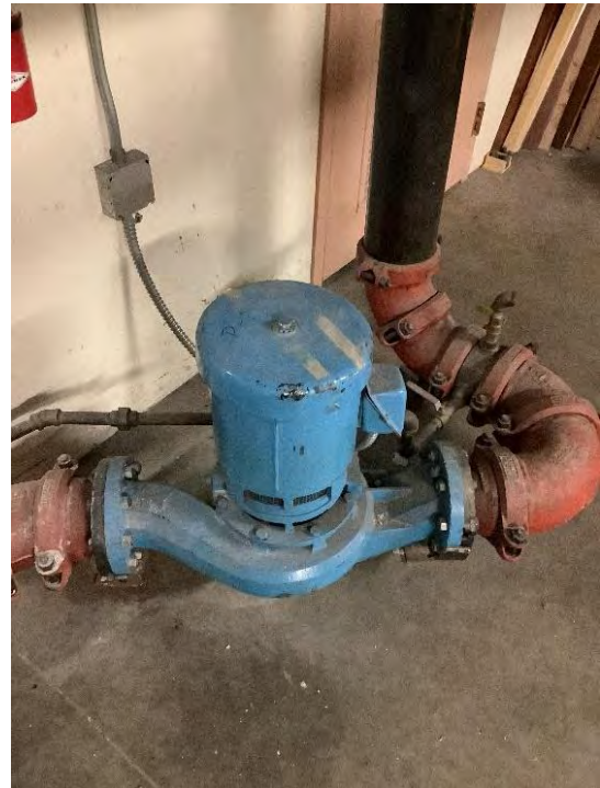
Fig 9: Chilled Water Pump-5
