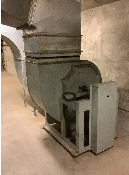
Fig 10: EF- North Switchgear Room
