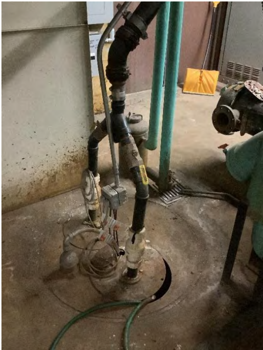
Fig 13: Sump Pump - 3 Basement 1966 Mechanical Room
