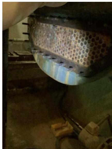
Fig. 5: Chiller-2 tubes exposed
