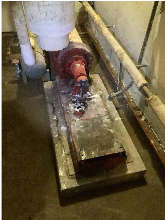
Fig 8: Chilled Water Pump 28-1-2
