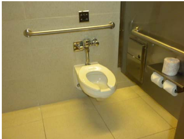
Photo 3: Automatic flush valve for toilet
