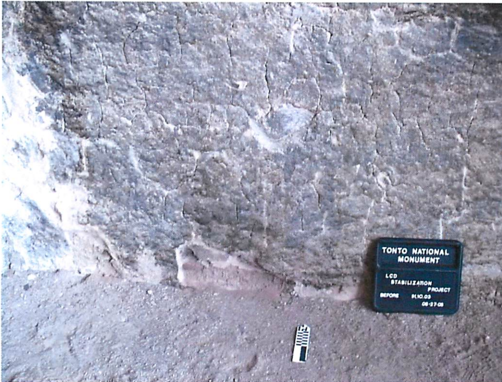
Figure 6. Before photo of wall 51.10.03.
